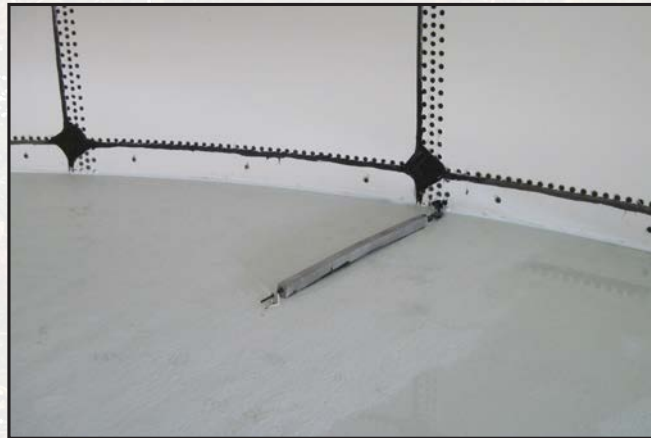
Anode on tank floor
