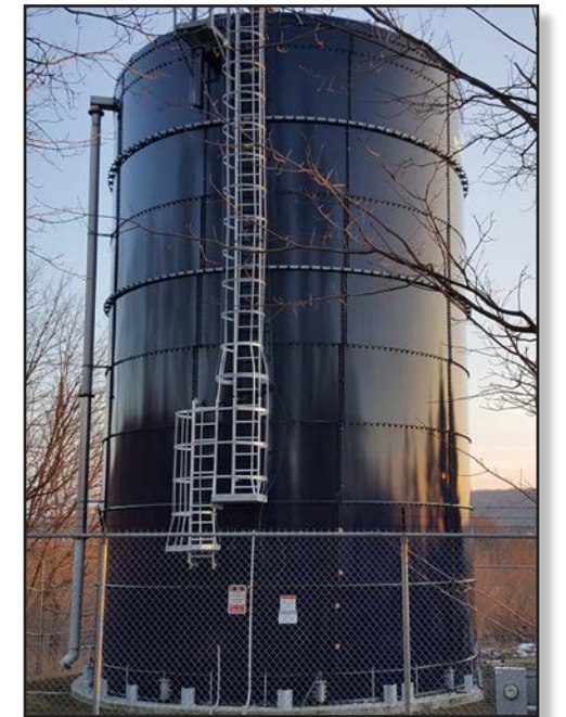
18yrs after original construction, there is no discernible difference between the original panels and the newly installed ones
