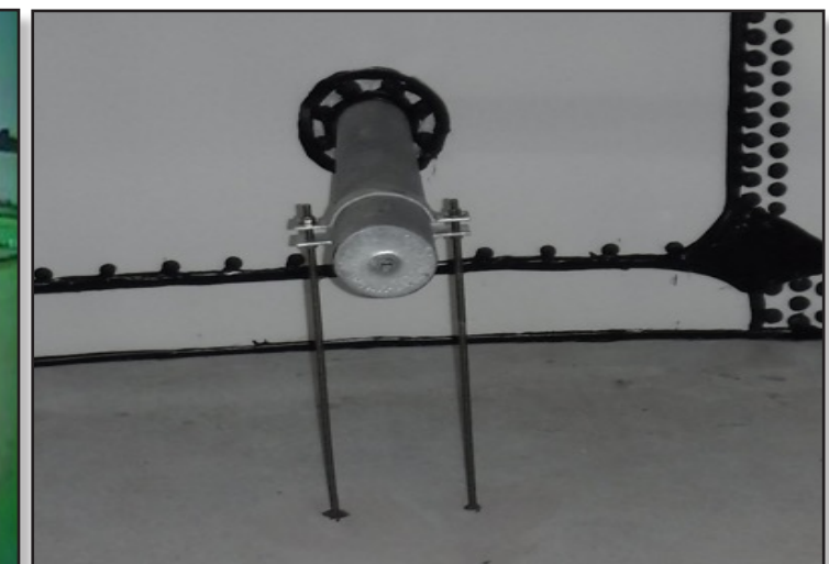
Heater, interior view
