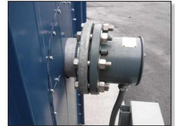
Heater with insulation on tank exterior
